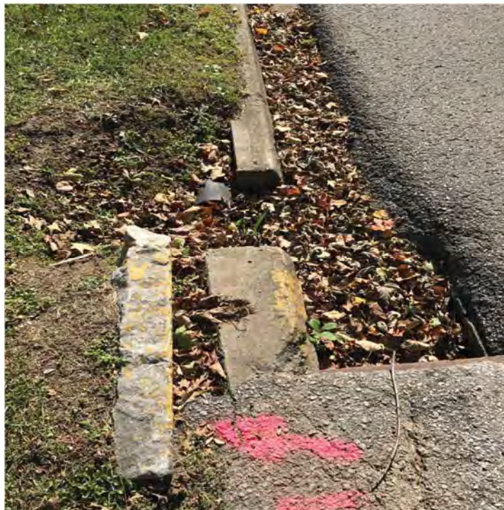
12. Looking south at stone and concrete curbs and gutter by street 600 block of N. Main in HD
