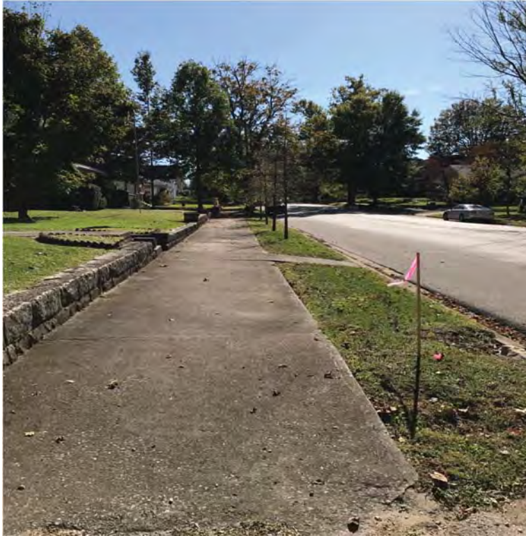
11. Looking south at sidewalk and retaining wall east side of 600 block North Main
